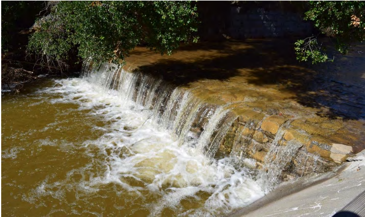
Figure 16. This check dam on Maria Ygnacio Creek below the UPRR bridge inhibits steelhead migration. February 6, 2019.
