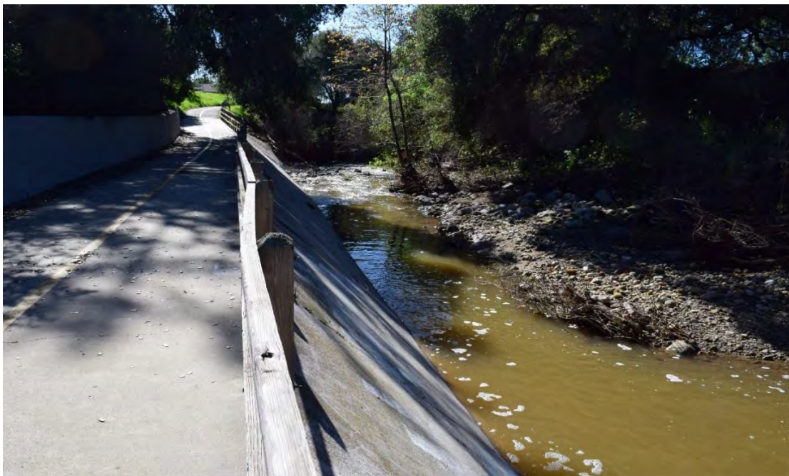
Figure 19. The Maria Ygnacio Creek Bike Path gives the public an up-close look at the Creek, but it also encroaches into the Creek habitat. Brian Trautwein. 2017.
