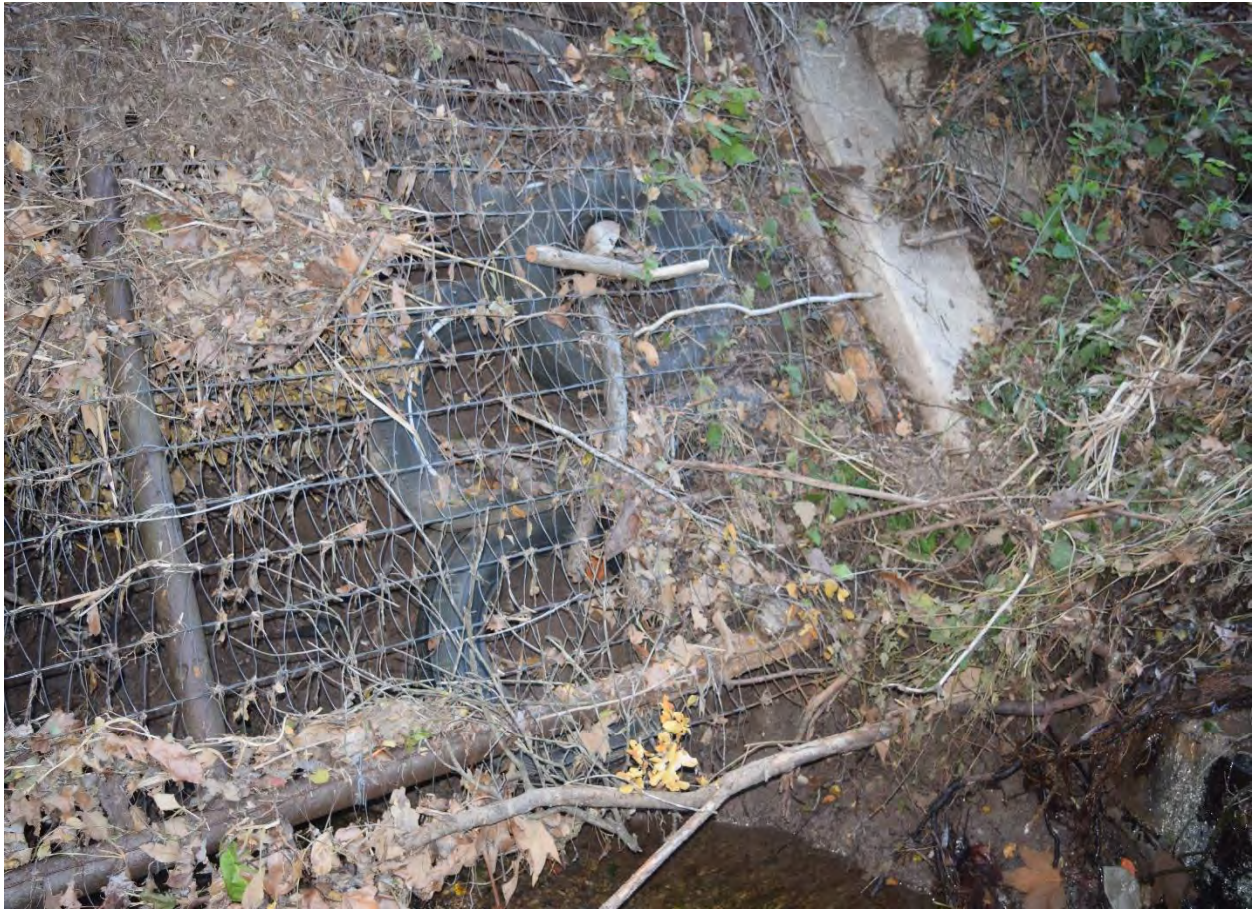
Figure 131. Old tires stacked behind pipe and wire revetment on west bank of San Pedro Creek downstream from Cathedral Oaks Road. Brian Trautwein. 2019.
