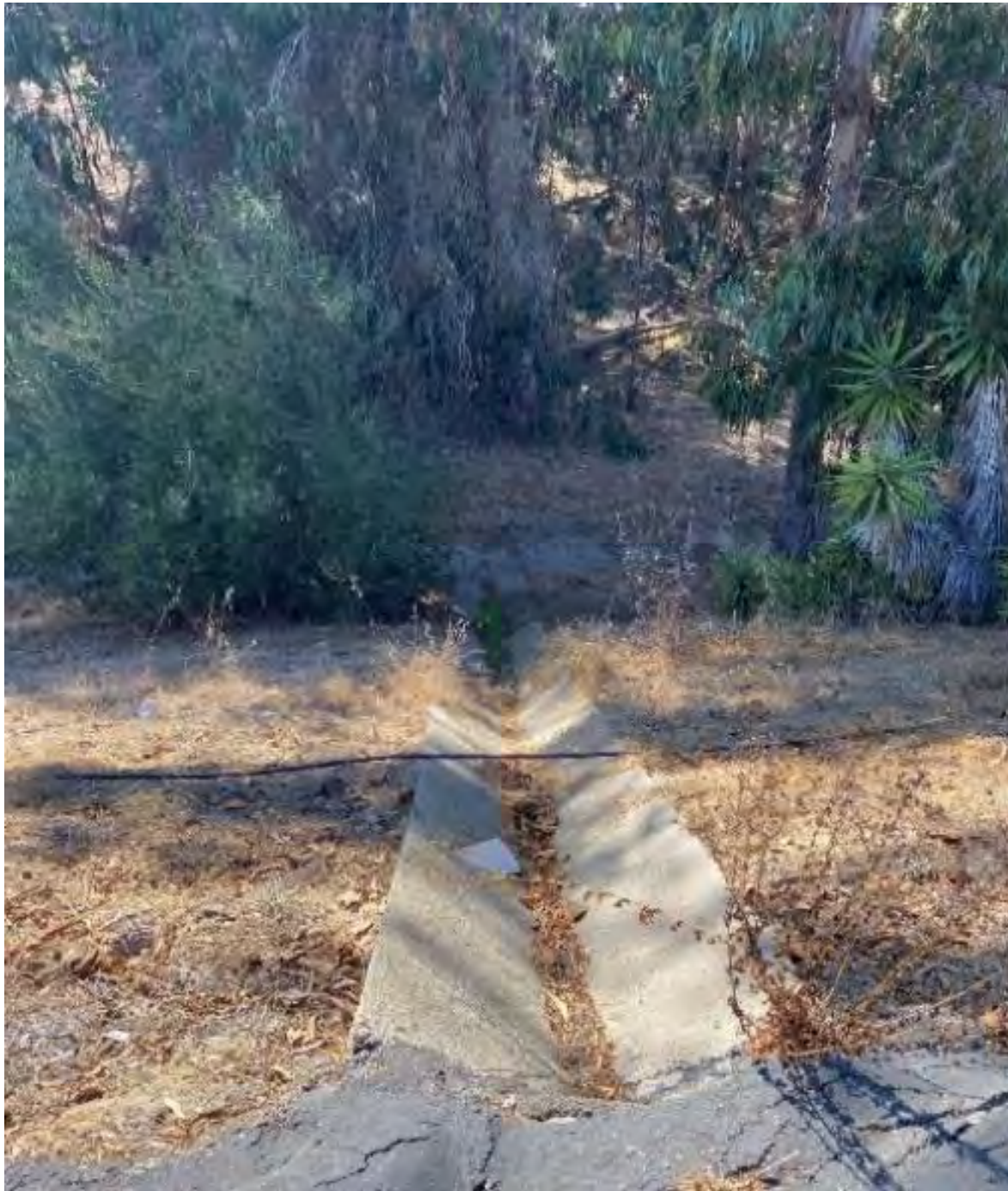
Figure 74. A concrete-lined storm drain directs parking lot runoff into the tributary without any opportunity for infiltration. Brian Trautwein. October 2020.
