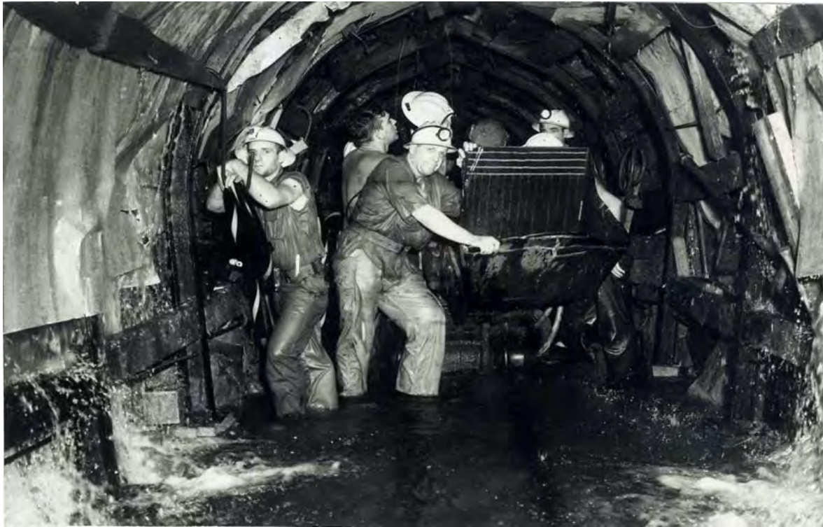
Figure 9. Workers constructing Tecolote Tunnel with groundwater infiltrating the borehole. Cachuma Operations and Maintenance Board, 1954.
